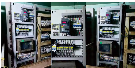
Material Cart Control System Application
